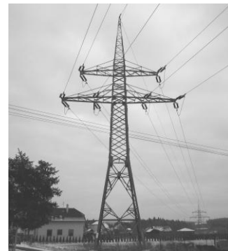
Fig. 1: Deviation tower with two parallel 110 kV overhead lines
