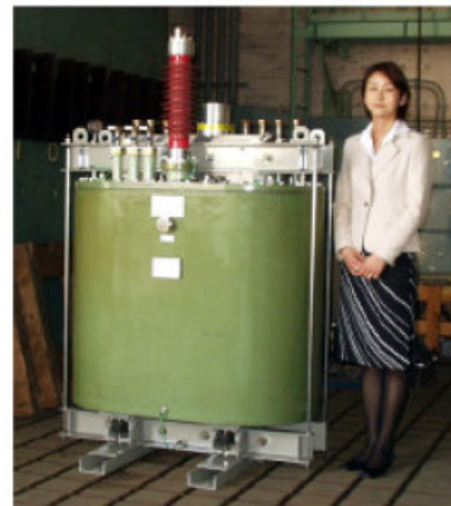
Fig. 1. 4MVA HTS transformer
