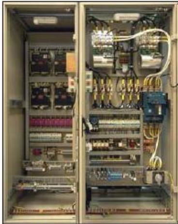
Part of PRISMIC® A50 excitation system for a 259MVA turbogenerator
