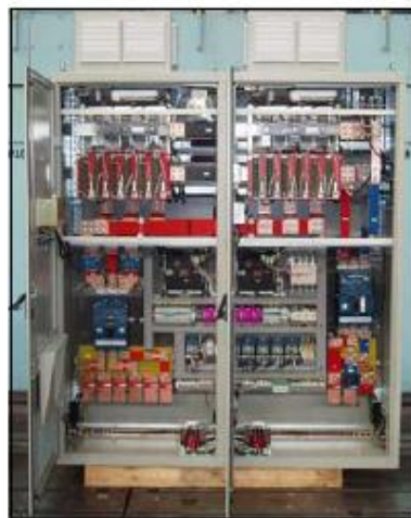
A BRUSH excitation system utilising modular power converters for a 140MVA turbogenerator
